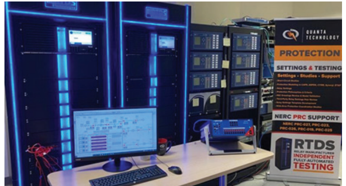
PICTURED: HIL test setup for FP&L project
