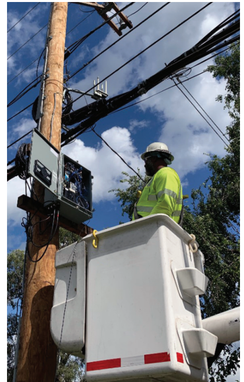
PICTURED: A SIMPLE device installed on a distribution pole along with radio
