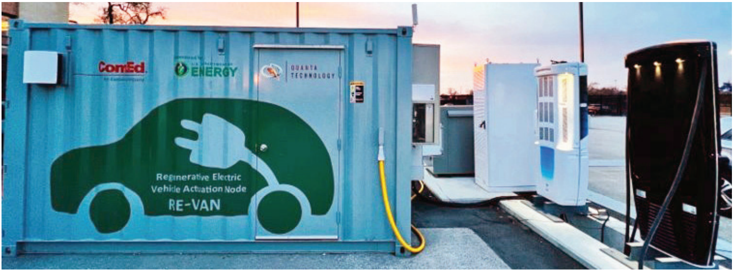
PICTURED: Outdoor lab setup for functionality testing dc fast and ultra-fast charging stations (up to 350 kW)
