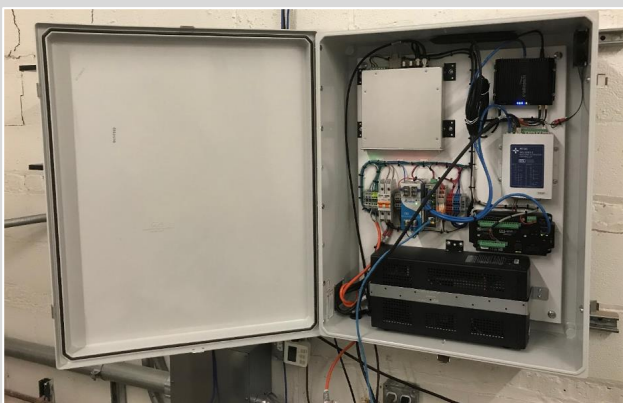
Site Controller and DER Aggregator
